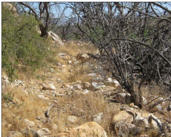
Looking down canal at the narrow, nearly completely filled channel of the Robinson Canal as it courses along the steep side of a mesa on its way to fields on Robinson Flat. Note the illusion of the canal coursing upslope.
